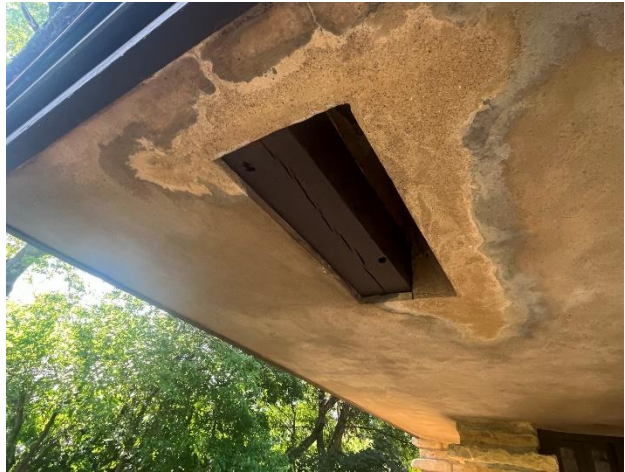
Figure 333. Previous stucco patch.
