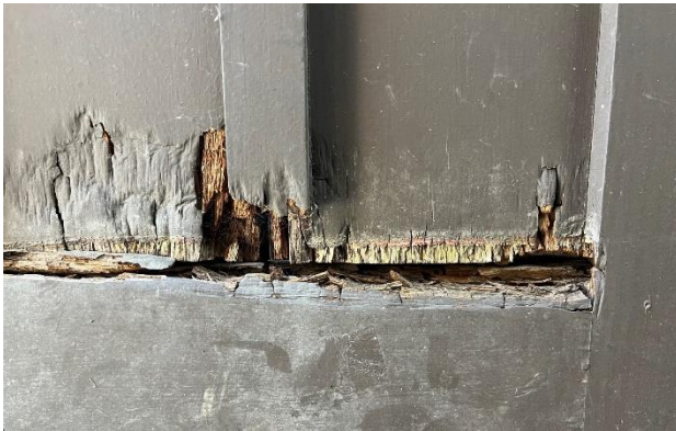
Figure 337. Distress at bottom end of door panels.
