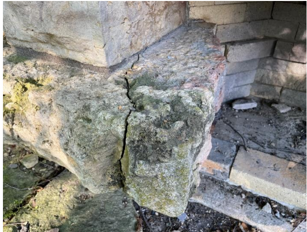
Figure 320. Cracked stone unit adjacent to steel lintel.
