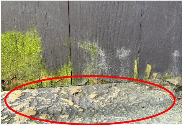
Figure 215. Isolated areas of peeling paint.
