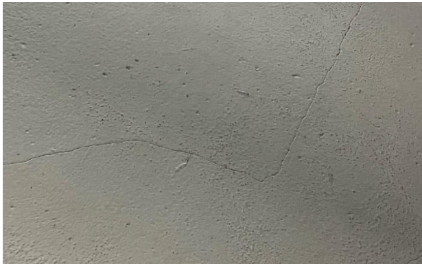
Figure 204. Incrementally stepped cracking across the plaster surface.
