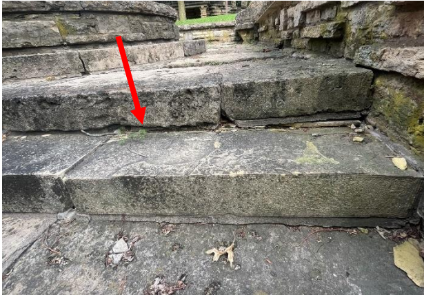
Figure 68. Open mortar joints at stone stair treads.
