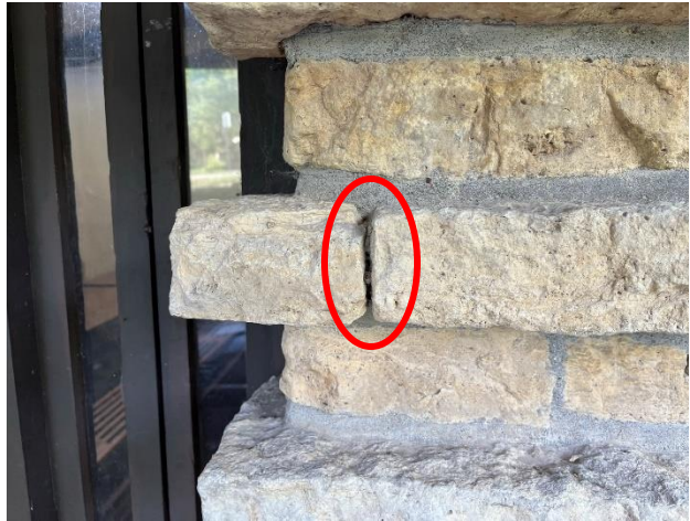
Figure 304. Open horizontal mortar joint.
