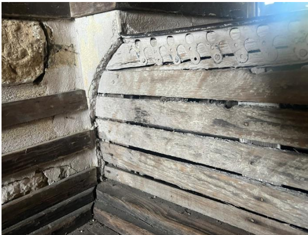
Figure 206. Exposed wood lath and edge beads.
