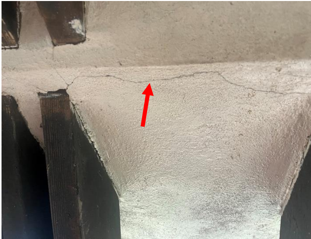
Figure 325. Hairline crack extending perpendicular between roof rafters.
