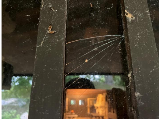
Figure 519. Cracked glass light at door.
