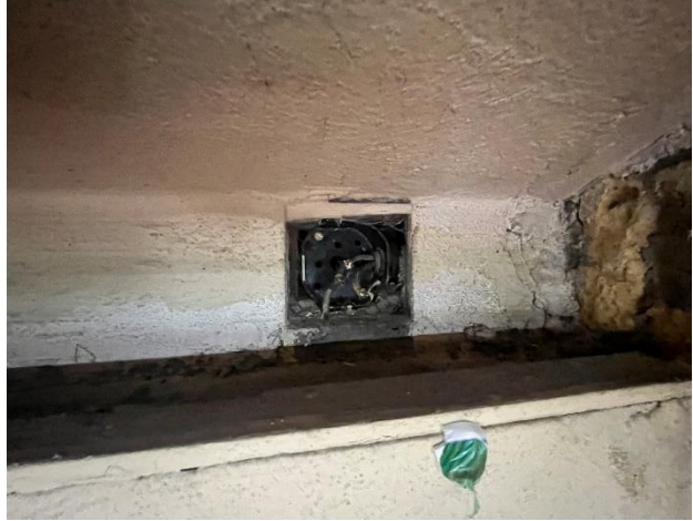
Figure 278. Cloth-jacketed electrical wire within the junction box.
