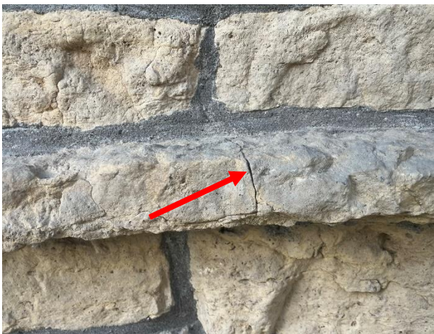
Figure 295. Crack running vertically through the stone.
