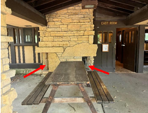
Figure 418. Two exterior fireboxes, one at each corner.
