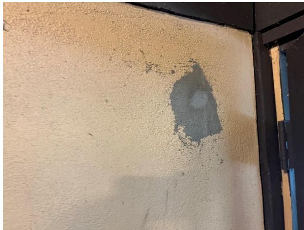
Figure 512. Unpainted patch at previous patch repair.
