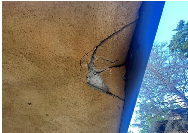
Figure 331. Cracked stucco with scratch coat exposed.
