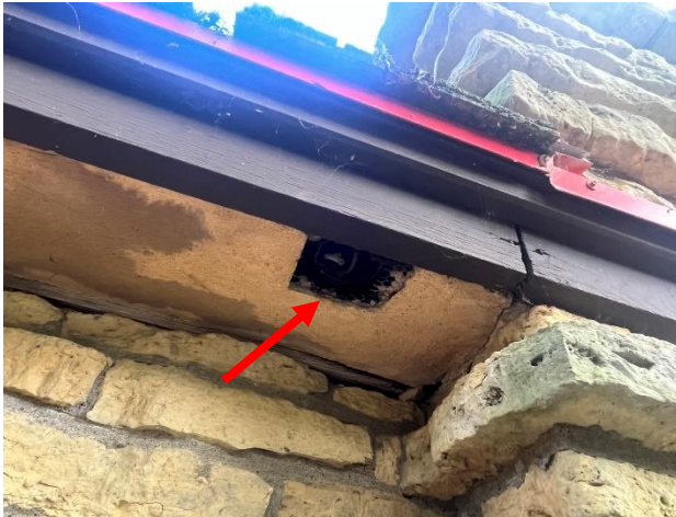
Figure 332. 7-inch square opening in stucco eave.
