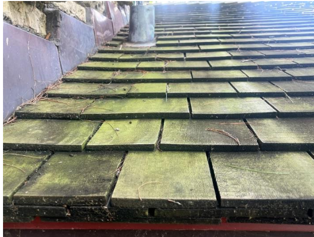
Figure 201. Biological growth at wood shingles.
