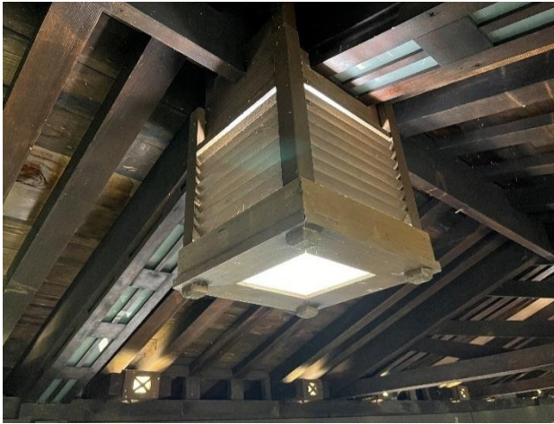
Figure 439. Lantern-style light fixture mounted to ceiling framing.
