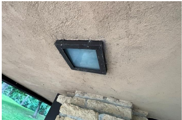
Figure 357. Recessed light fixtures in the soffit.
