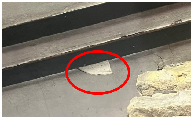
Figure 205. Debonded plaster finish that has fallen loose.
