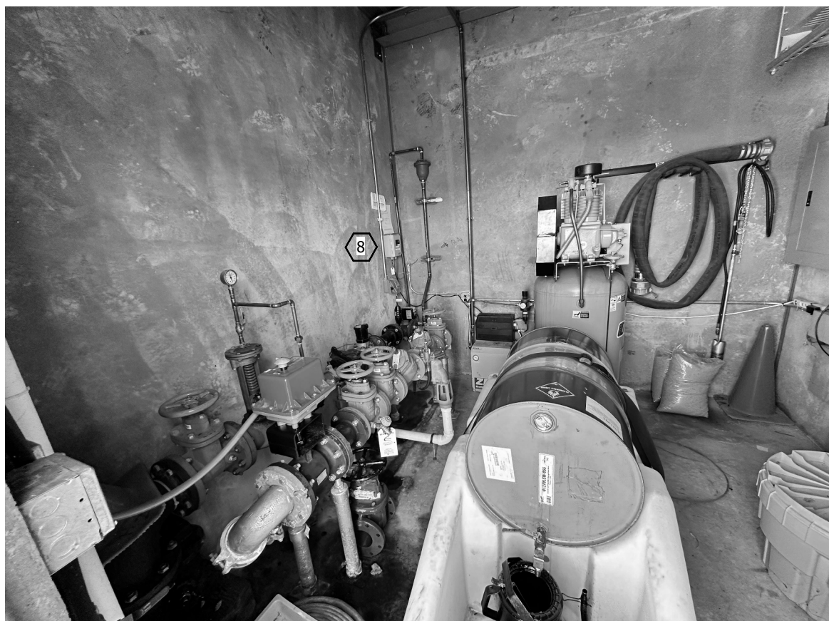
EX WATER SERVICE ENTRANCE IN PUMP HOUSE
